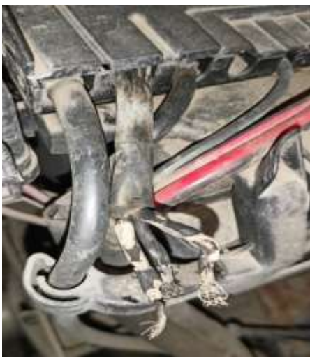
Fig. 2. Damaged - burnt electrical insulation
