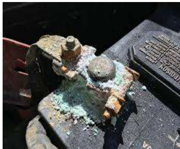
Fig. 3. Oxidized electrical connections
