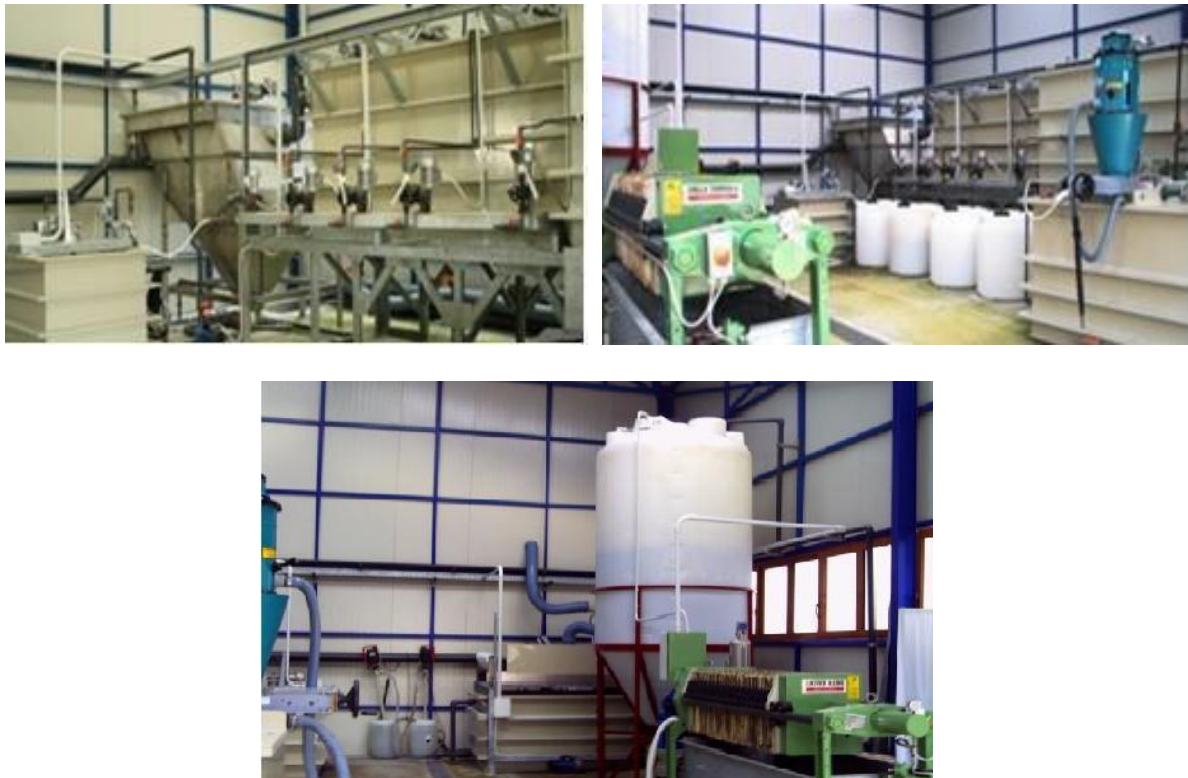
Fig. 2. View of the plants for primary and secondary treatment of bilge water
