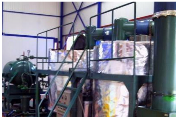
Fig. 3. Depuration plant for cleaning waste
