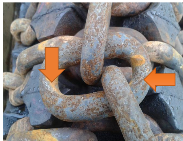
Fig. 6. Visible areas of abrasive wear in the area of the link joint
