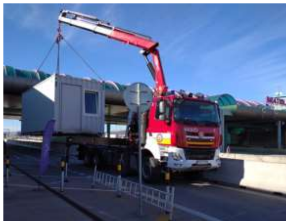
Fig. 4. Installation of an administrative container at the border crossing point of Jarovce - Kittsee [1]
