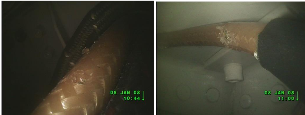
Fig. 5. Chafing between two adjacent cables due to insufficient separation
